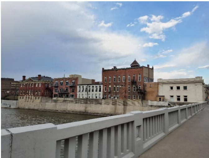
Figure 59: The river wall located north of Main Street, looking northeast from the Main Street Bridge (ASI 2021).
