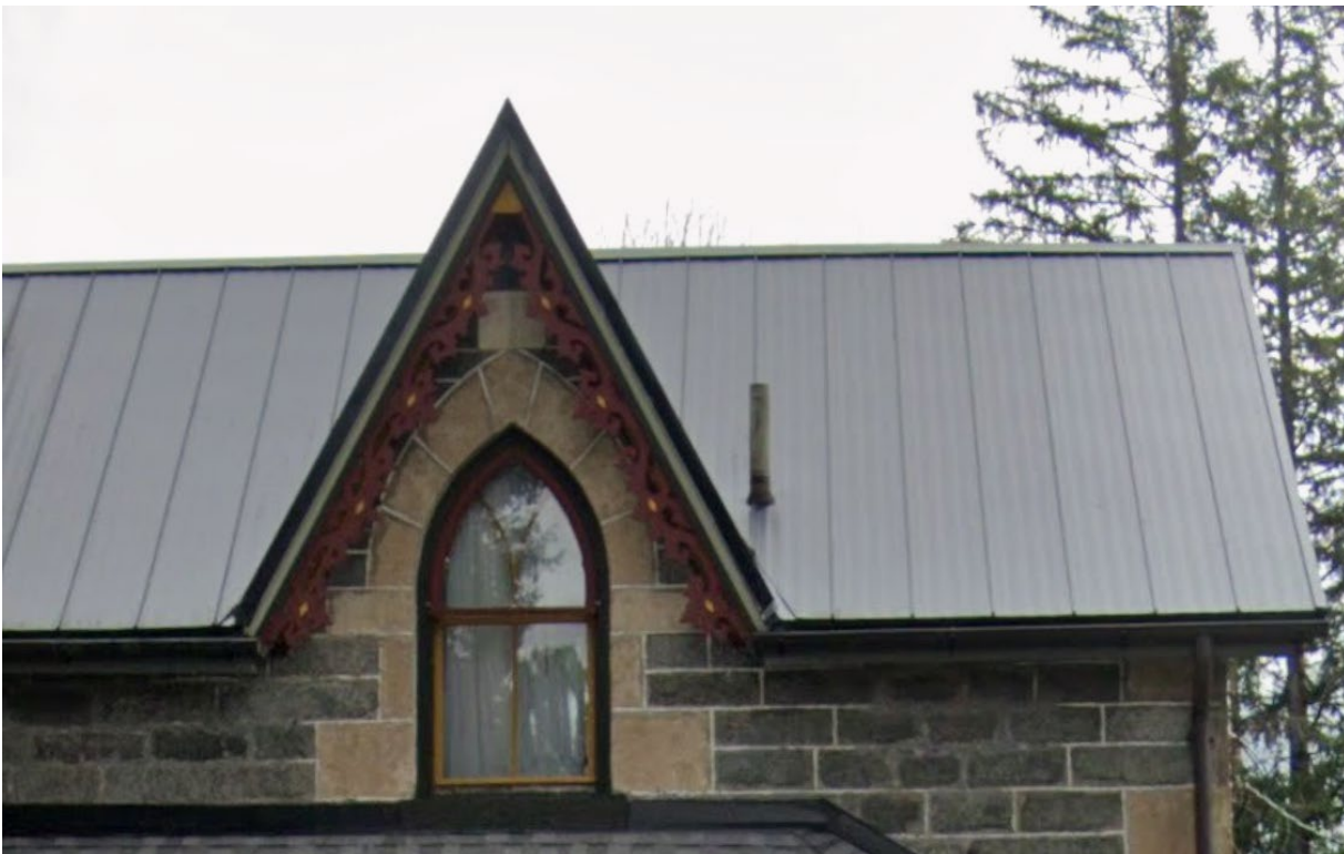
Figure 2 – Close up picture of the roof peak sills and details at 77 Lowell Street North taken from Google Street View, September 2022
