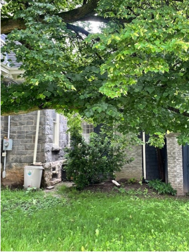
Figure 5: Rear elevation showing the single-storey shed-like addition, constructed in materials and finishes consistent with the original granite masonry.
