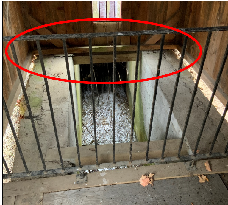
Photograph 10: Spalling concrete at cast-in wood
