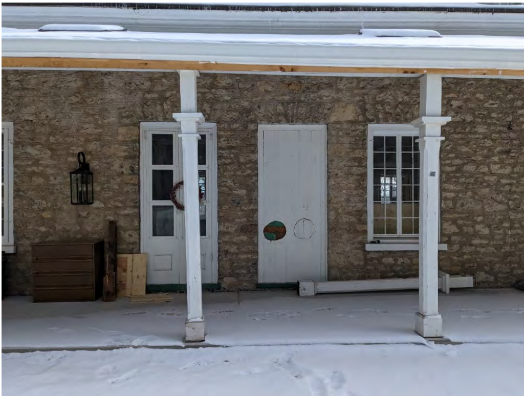
Figure 18: Green wooden floor no longer present, west elevation
