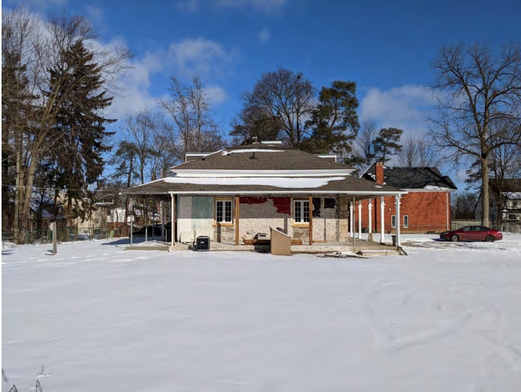
Figure 13: View north of south elevation where the kitchen and bathroom have been removed
