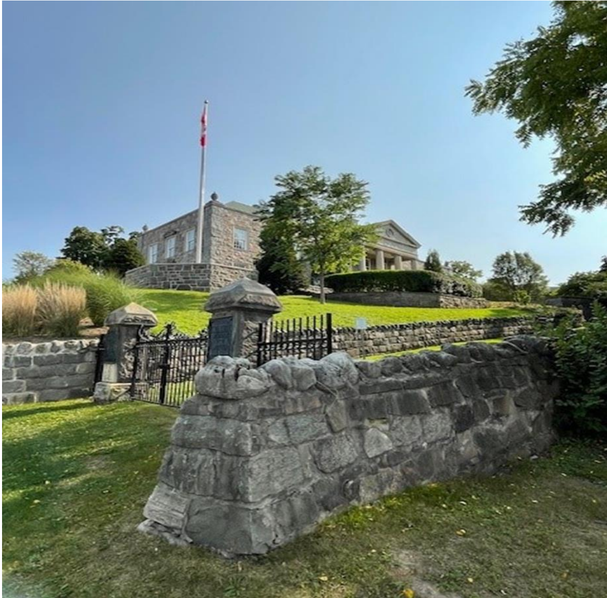
Figure 2: A section of the stone retaining wall along Dundas Street North (Scott Abbott, City of Cambridge).
